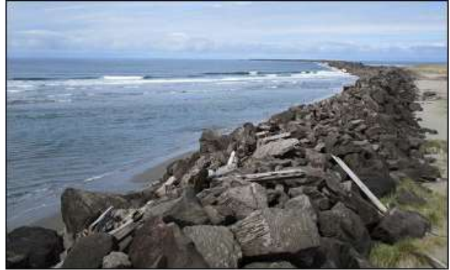
This breakwater separates the Columbia River from the ocean in nearby Fort Stevens. Photo by Rick Hull
